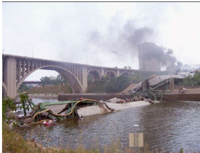
Figure 2 – Minneapolis Bridge After Collapse
